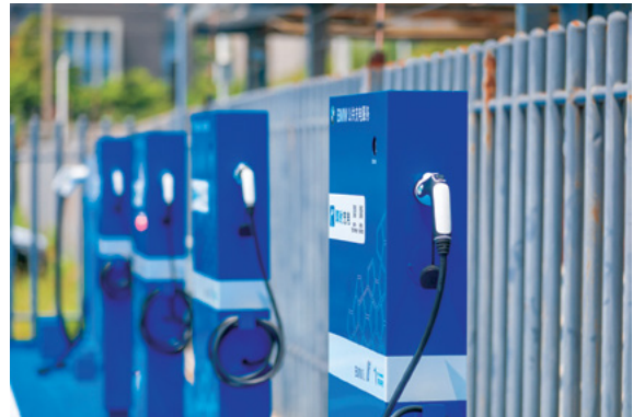
ChargeNow charging pillar.
