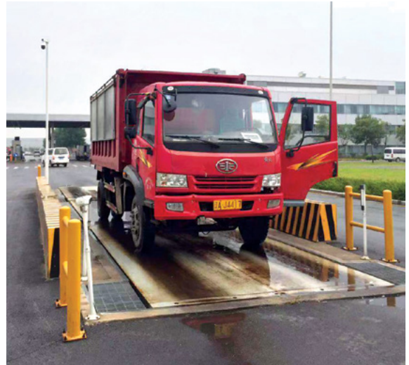
Newly installed waste weighing system.
